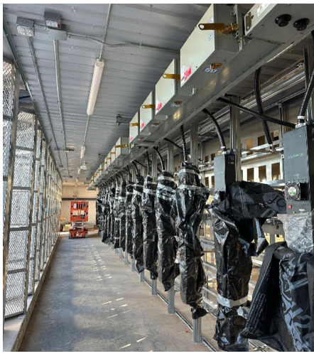
Childress – data center internal electrical fit out
