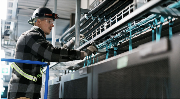
Prince George Data Center (August 2025)
