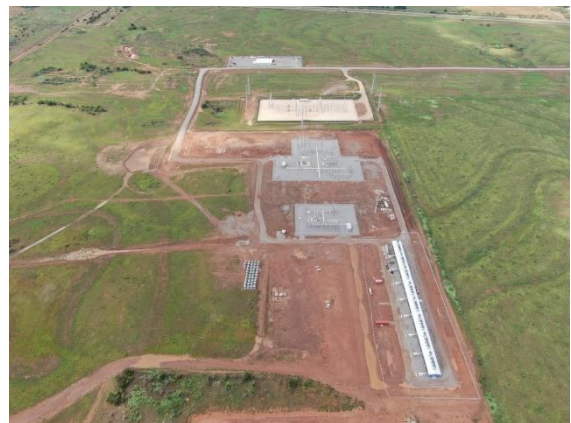
Childress – aerial view of the 600MW site
