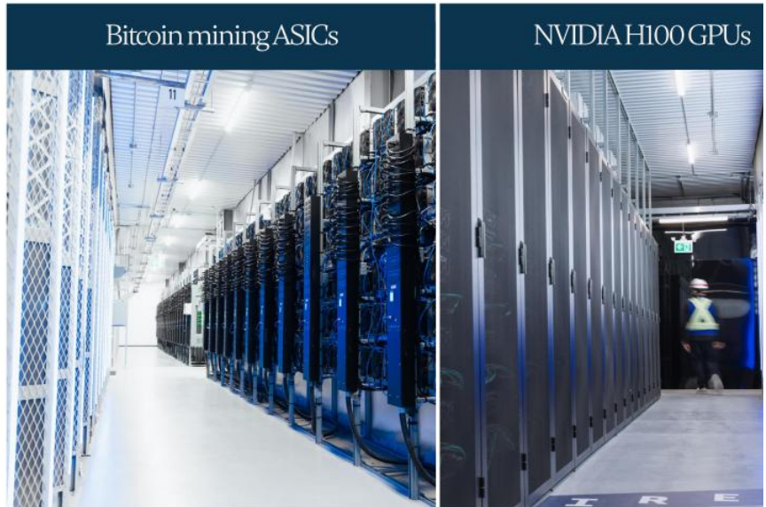
Prince George Data Center ASICs & GPUs
