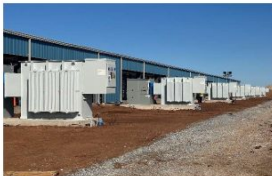
Childress – DC 2 electrical installation
