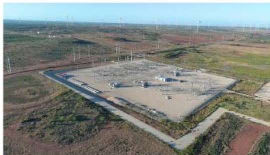
Sweetwater Utility Substation
