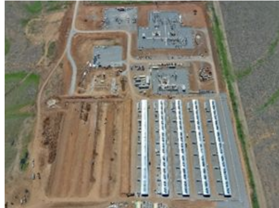
Childress (March 2024) Expansion to 100MW in H1 2024 nearing completion Expansion to 300MW in H2 2024 underway
