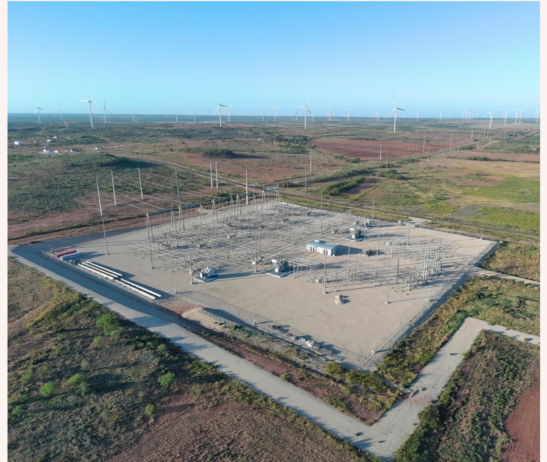
Existing utility substation adjacent to Sweetwater site
