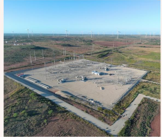
Existing utility substation adjacent to Sweetwater site
