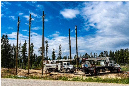
Mackenzie – high voltage tap connection
