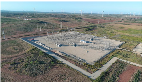
Sweetwater Utility Substation
