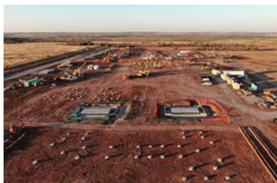
Childress – aerial view of the construction of the 600MW substation and first data center building (20MW)
