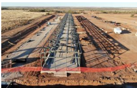
Childress – aerial view of completed foundations and erection of structural steel for the first data center building (20MW)
