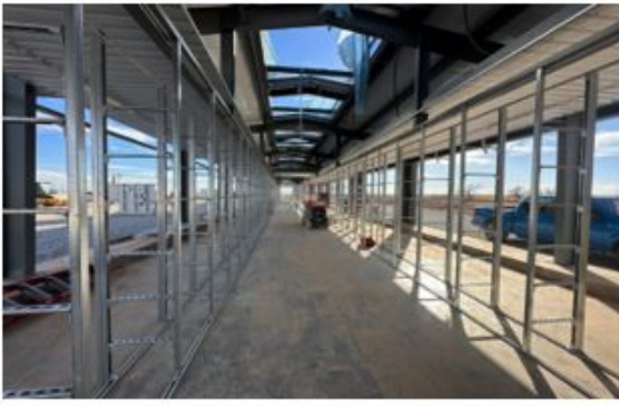
Childress – internal fit out of miner racking for the first data center building (20MW)
