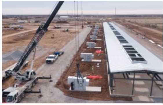
Childress – aerial view of low-voltage transformer installations at first data center building (20MW)
