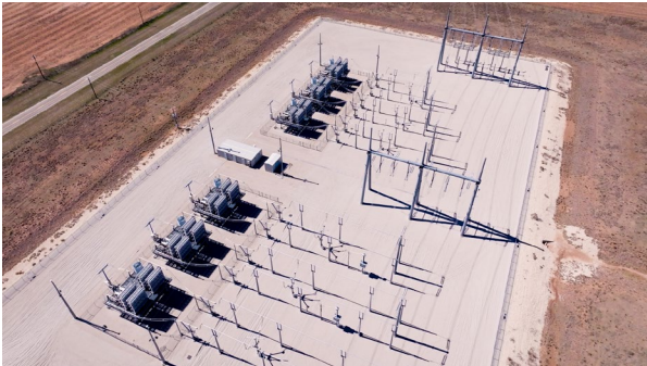
Utility Switchyard at Sweetwater 2 (Mar 2025)
