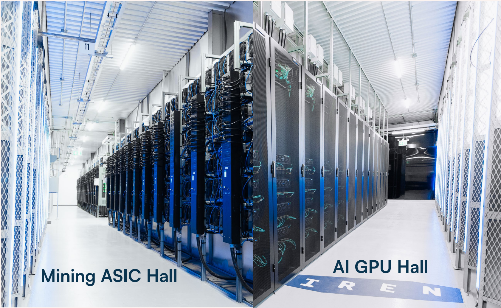
Prince George Data Center
