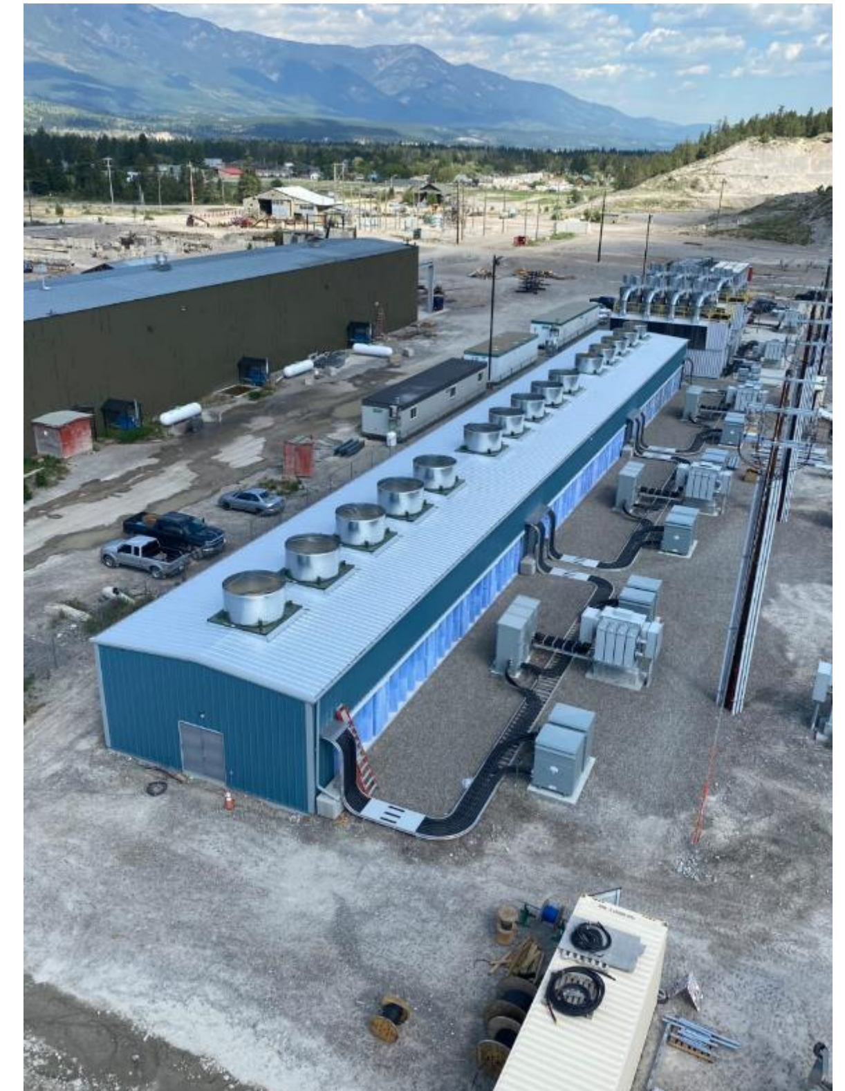
Existing data center at Canal Flats
