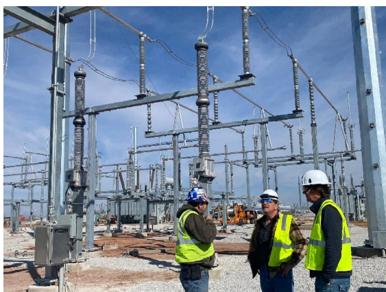
Childress – 345kV substation infrastructure
