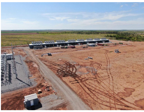
Childress – operational 20MW data center
