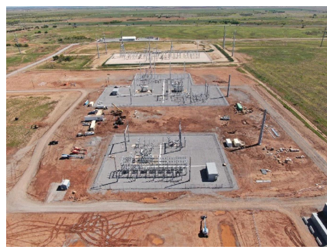
Childress – 600MW high voltage connection
