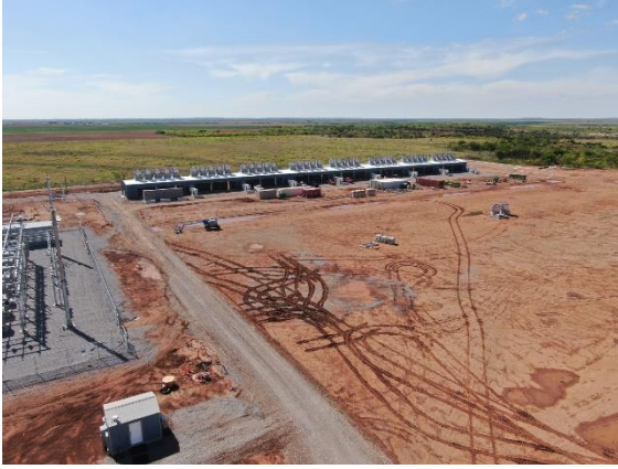
Childress – operational 20MW data center
