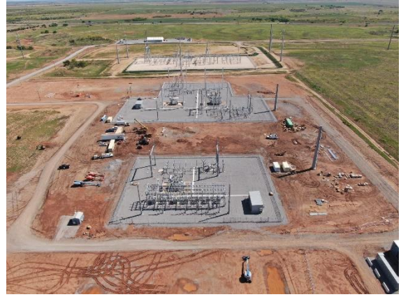
Childress – 600MW high voltage connection
