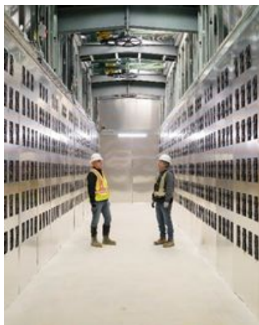
Mackenzie – miners installed in the first 20MW data center
